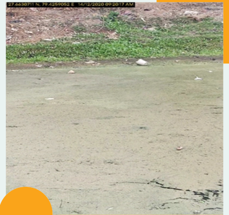
Waste on the surface UP_USMANPUR_110677_010461_W1
