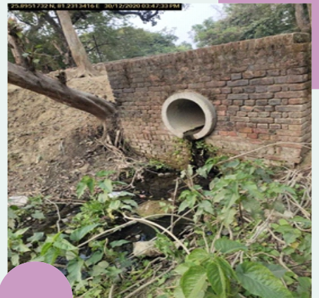
Drainage connected | UP_KHARALI MUSTAKIL_145240_009541_W1
