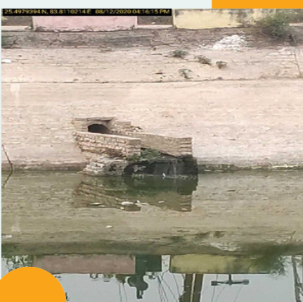
Drainage connected UP_GAHMAR_206711_006852_W2
