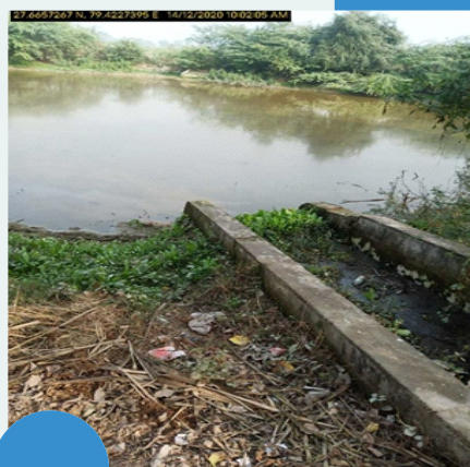
Drainage connected UP_USMANPUR_110677_010462_W2
