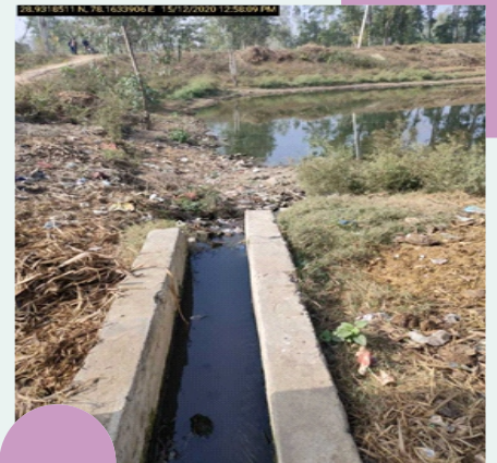
Drainage connected UP_WAJIDPUR_109641_008221_W1
